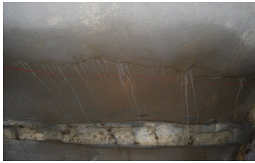
Figure 3: Seepage water draining into pipeline
