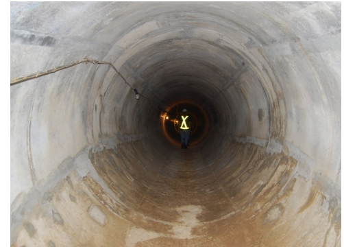
Figure 4: Initial interior surface conditions of the pipeline
