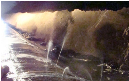
Figure 2: Leaking after conventional crack sealing
